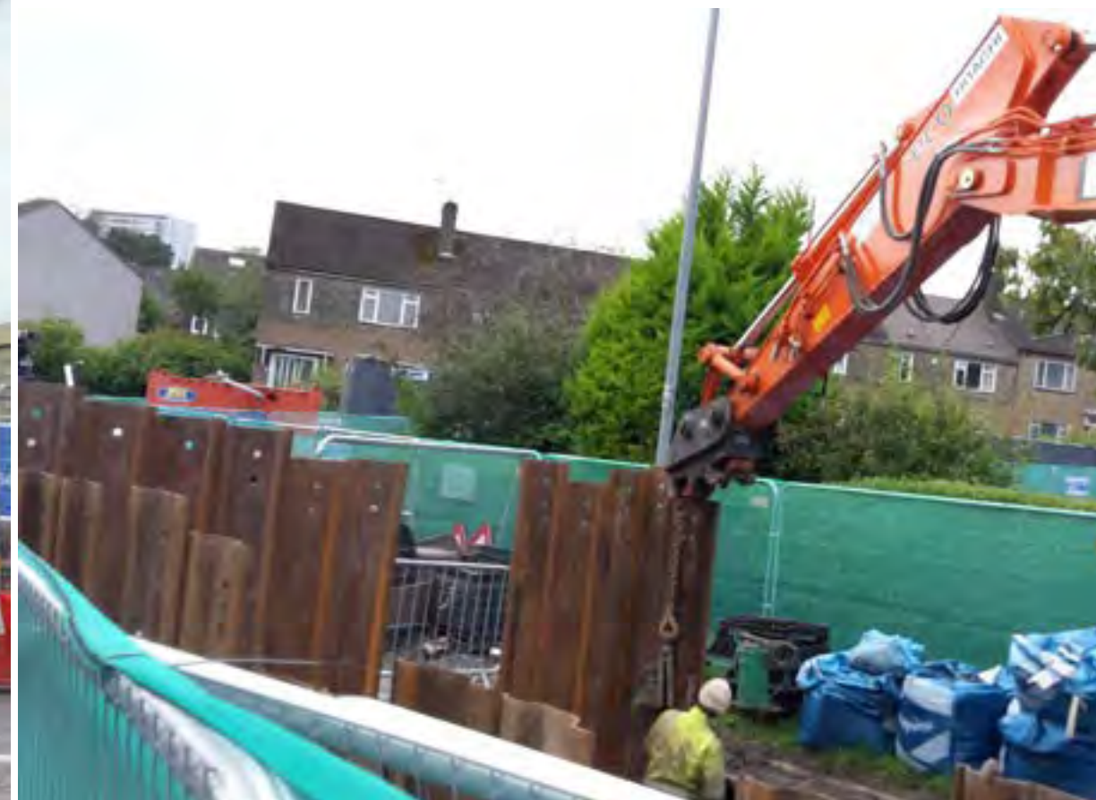
4) To install the large pipes, the ground is firstly secured by piling metal sheets into the ground. This phase can be noisy and cause vibrations.
