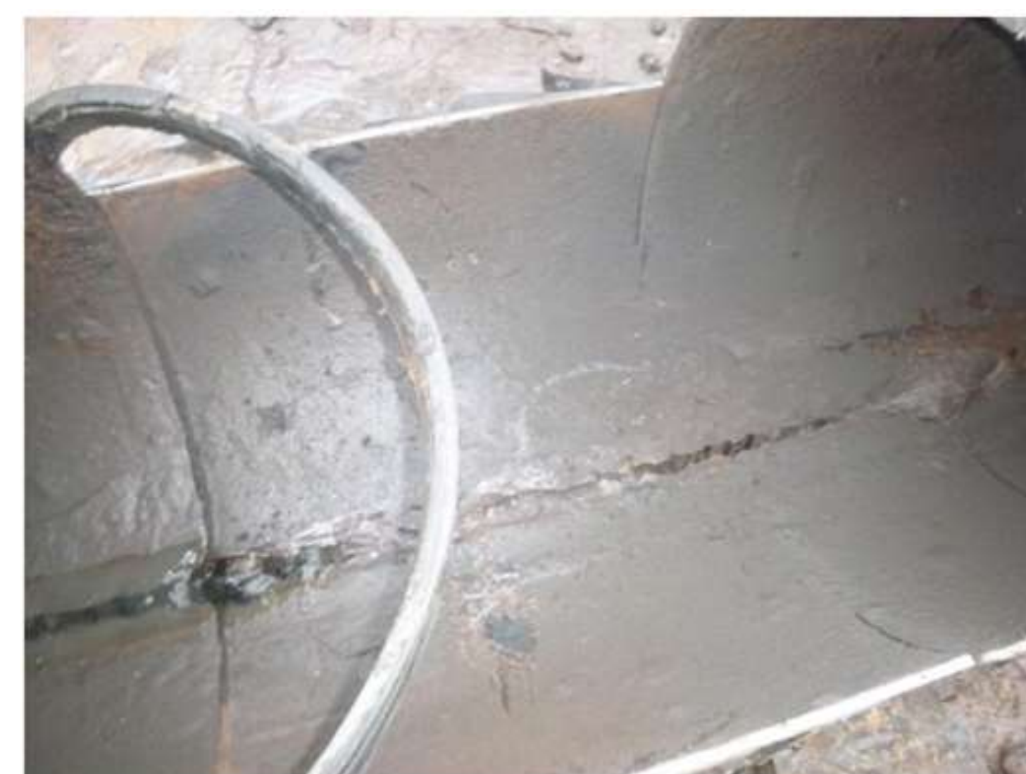
Showing Fracture along bottom of pipe
