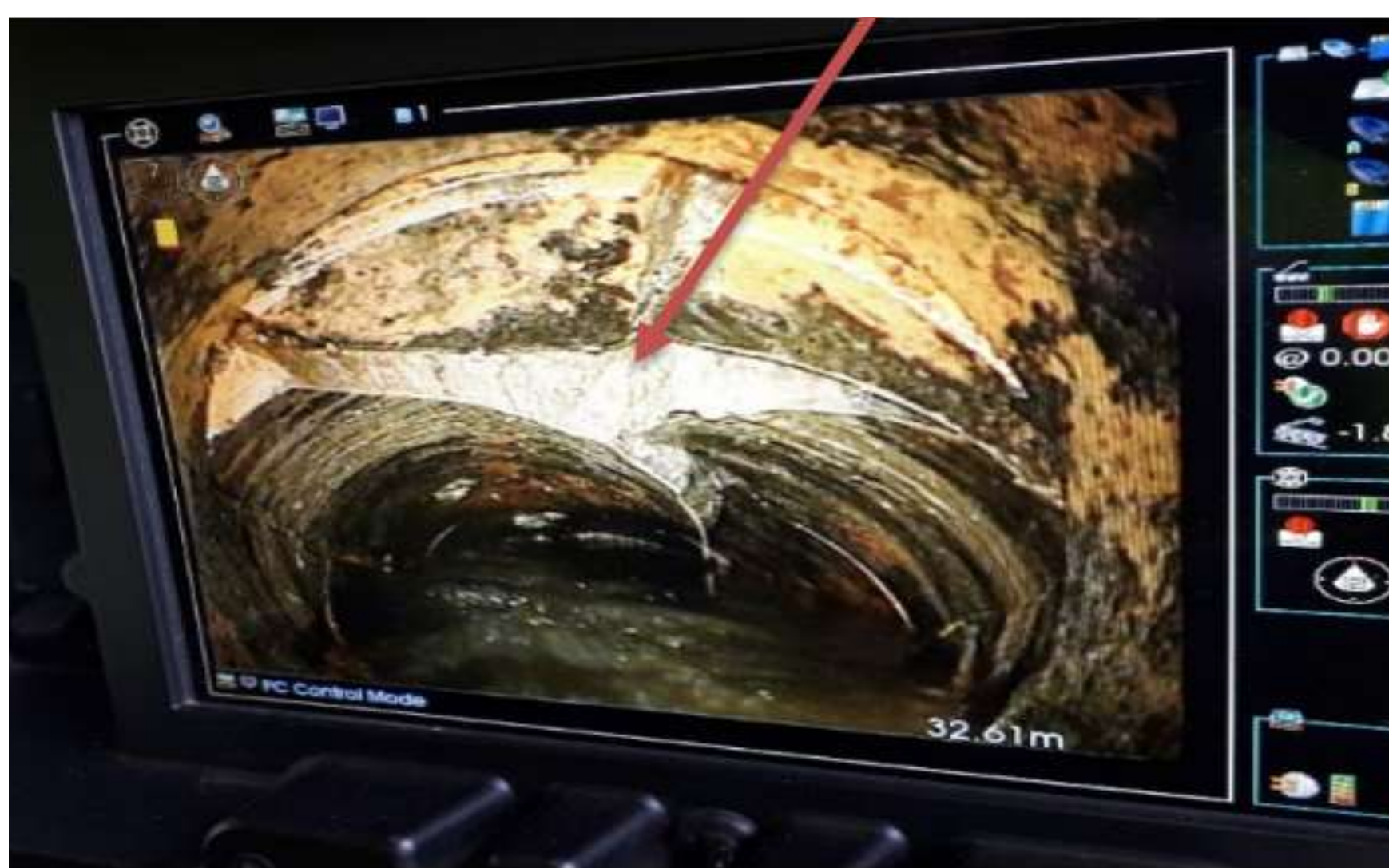
CCTV Survey image of the rising main
